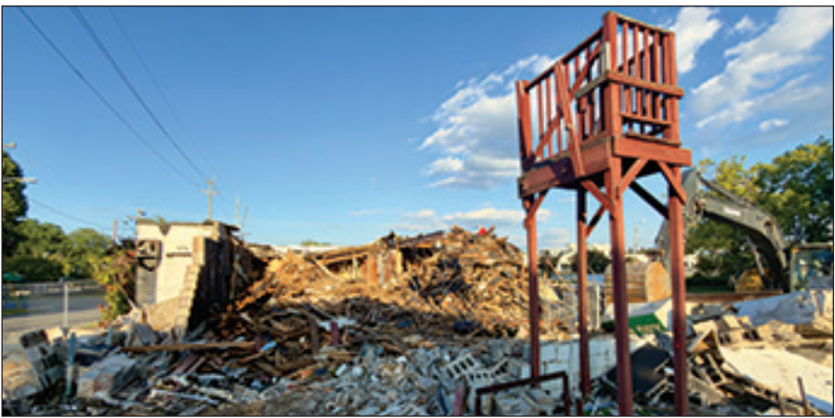
A wooden fire escape is the lone remaining piece of the Historic Excelsior Club on Beatties Ford Road after its July 15 demolition.
