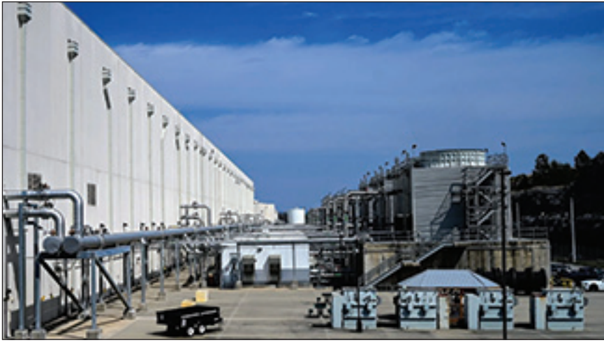
Cooling modules operate outside the Google data center in Lenoir, in Caldwell County. The facility was built in 2007 but announced a $1 billion expansion in 2026.
